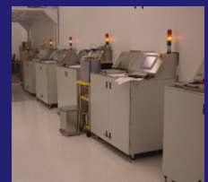
Process Services Available in both the U.S. and Japan. R&D and pilot production
