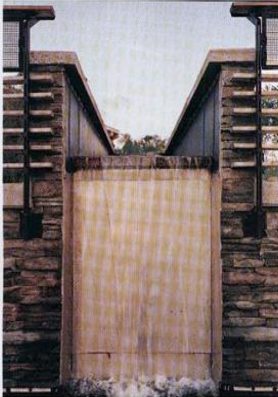
At the Discovery Health Center, rainwater flows into a trough (above), which is both an irrigation system and a holding tank for the fire-suppression system.
